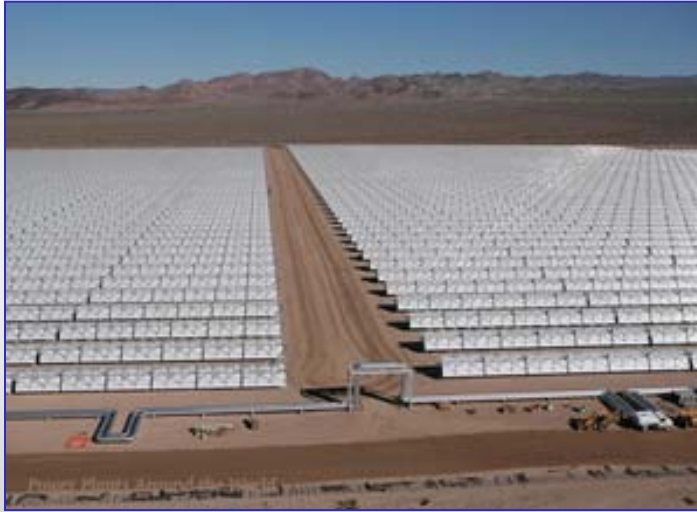
Nevada Solar One
