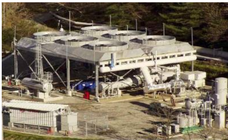
Fig. 3. Single-phase 2.2 MW Hatchobaru Plant in Japan
