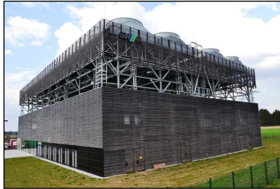
Figure 2. Sauerlach geothermal plant.
